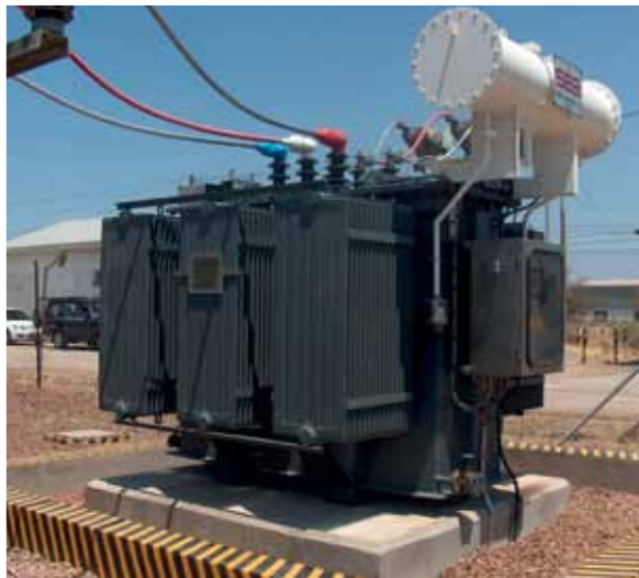
■ 10 MVar reactor in Botswana
