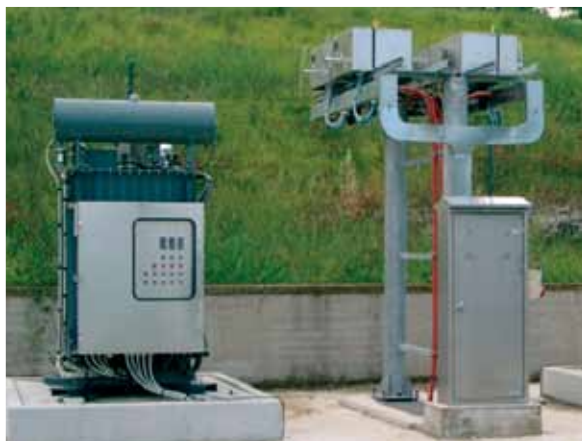
■ An example of Petersen Coil application
